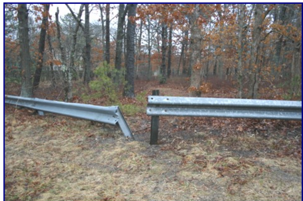
A vandalized guard rail on Pleasure Drive allows motor-bike access into the Flanders Pine Barrens.
