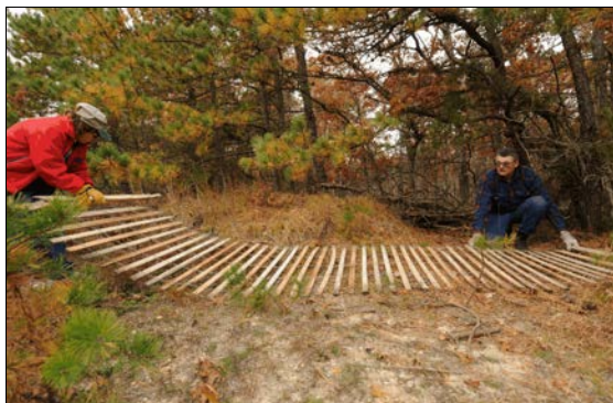
The LEC has supported the ATV Damage Mitigation Project in 2008, as on this November 5 th work day repairing barriers in the Flanders area.
