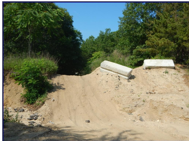
Damage and erosion caused by Illegal ATVs
